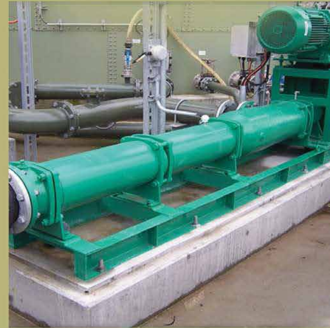
DIGESTATE TRANSFER PUMP Flow – 75 m 3 /hr, Pressure – 10 bar
