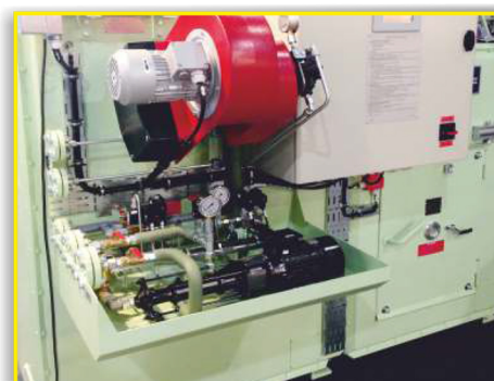
Roto Pump feeding dirty oil for incineration
